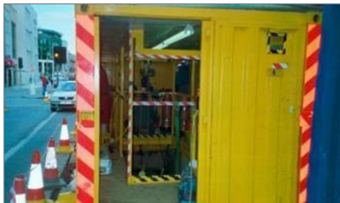
Figure 14 - HV cable jointing container
